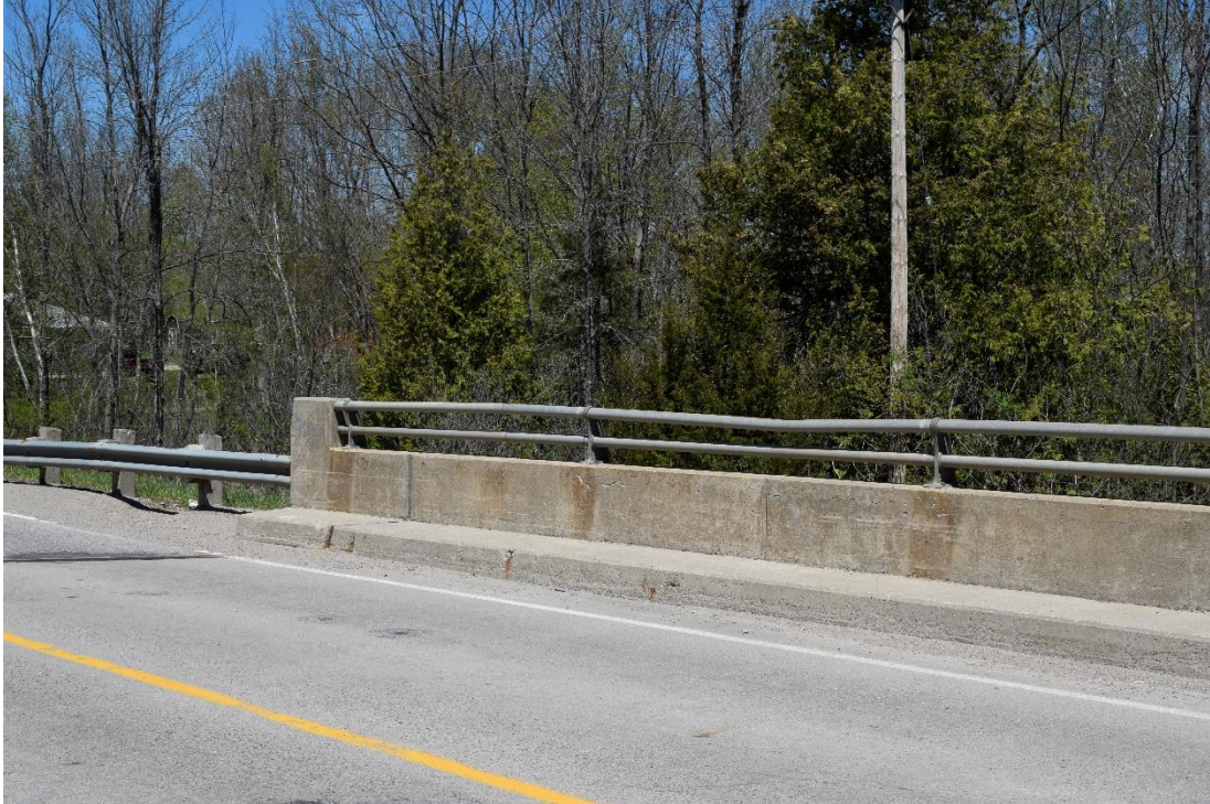
Image 5: Bridge parapet and guard rail note, deformation of railing, facing south
