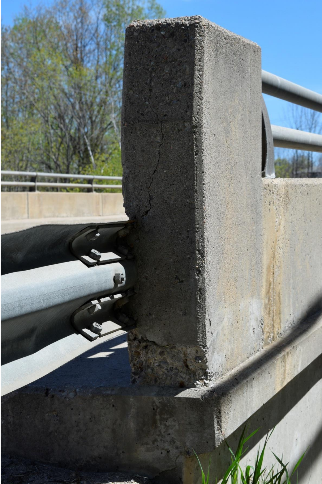
Image 7: Example of spalled concrete and water stains on bridge parapet wall
