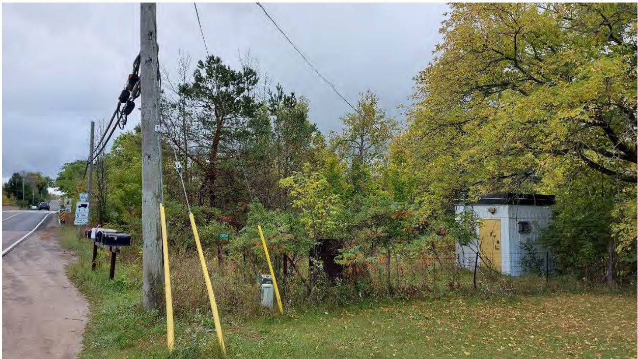
Photo 8: View of Bell telephone junction boxes located on the northwest side of the bridge, facing south.
