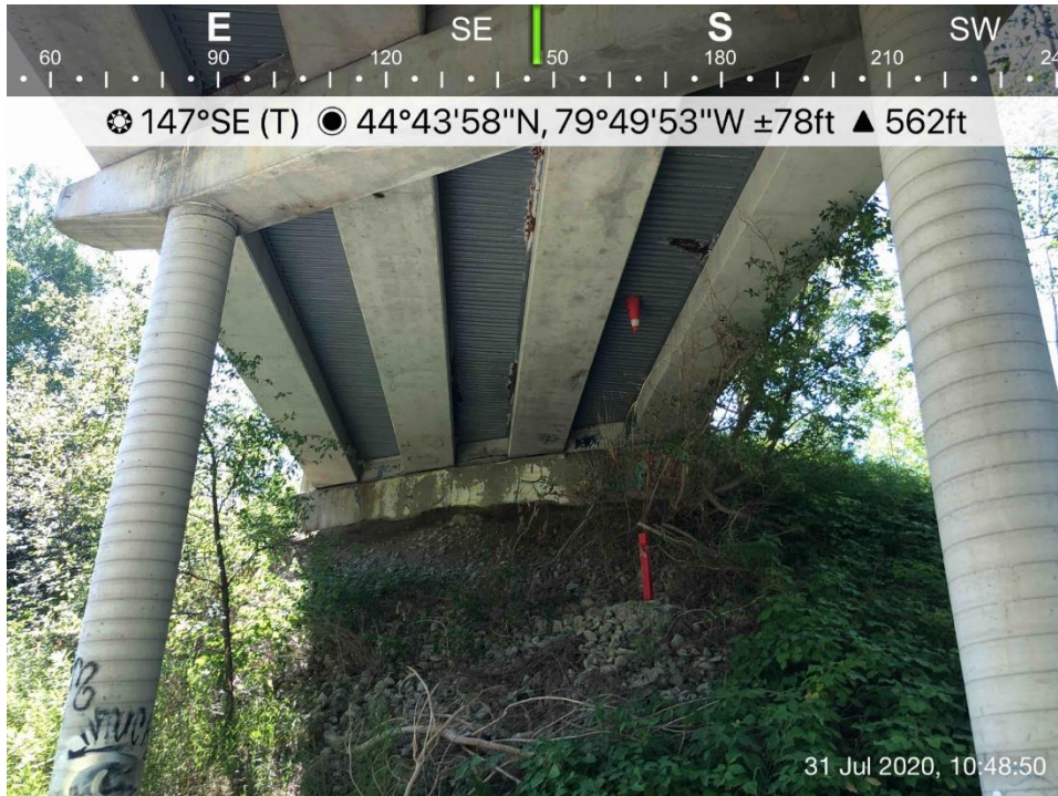
Photo 9: Photo taken under the north side of the bridge. No nests active or historical were observed. July 31, 2020.
