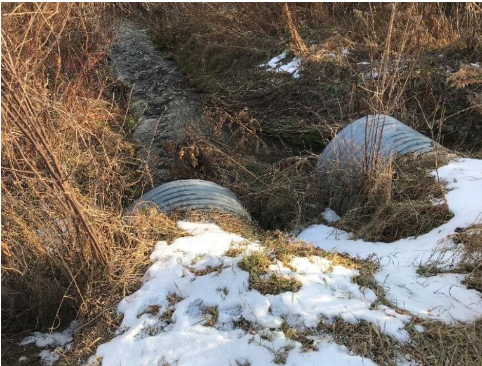
Image 11 Culvert under rail corridor; Channelized and culverted section of Warrington Creek tributary is disturbed, no potential
