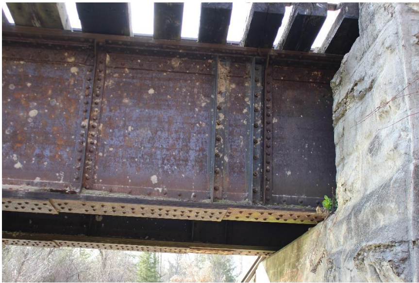
Plate 6: Detail of riveted plate girder, looking south with the west abutments at far right.
