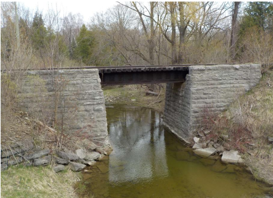
Plate 34: Barrie-Collingwood Railway Structure #3, Bateaux Road, Batteaux deck plate girder bridge (County of Simcoe n.d.)
