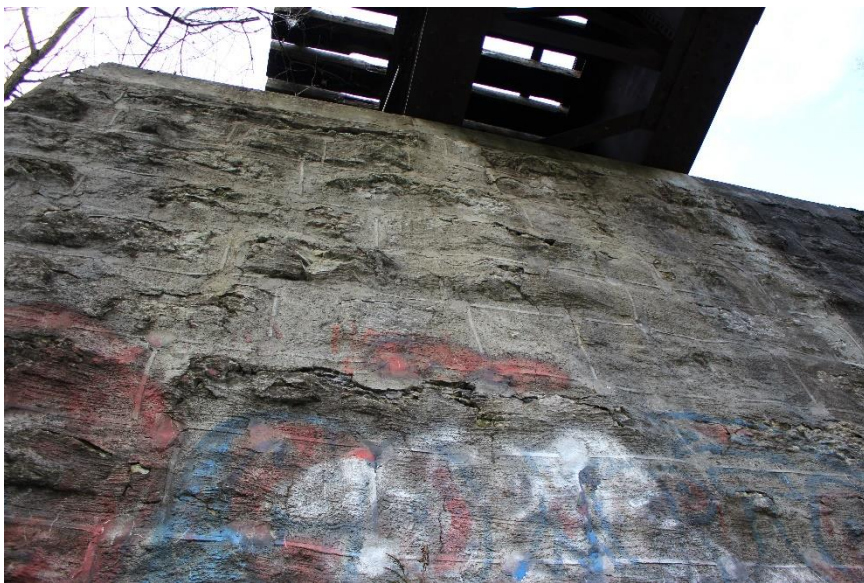
Plate 26: East face of the west abutments, showing deteriorated parging with score lines on the stone masonry, looking west.
