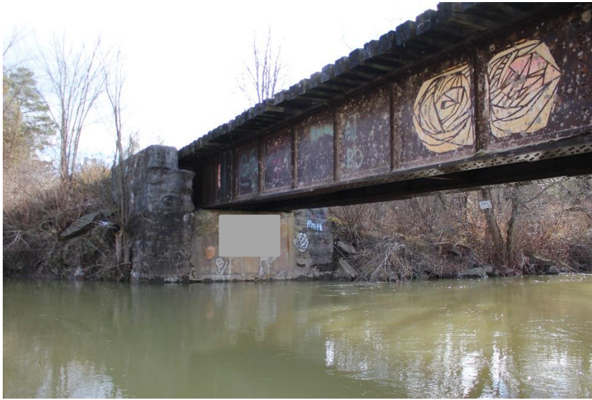
Plate 3: Oblique view of the north elevation and the east abutment, looking southeast. Note: the image has been altered by ASI to block offensive graffiti.
