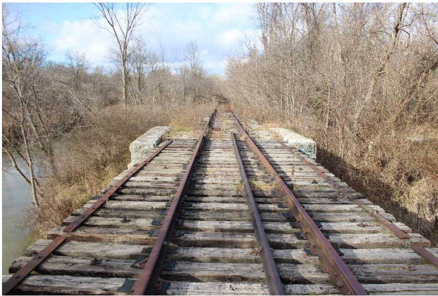
Plate 8: Open bridge deck with timber ties, rail track, and a single bridge rail, looking west towards the west approaches. Note the fallen tree blocking the rail track in the background.
