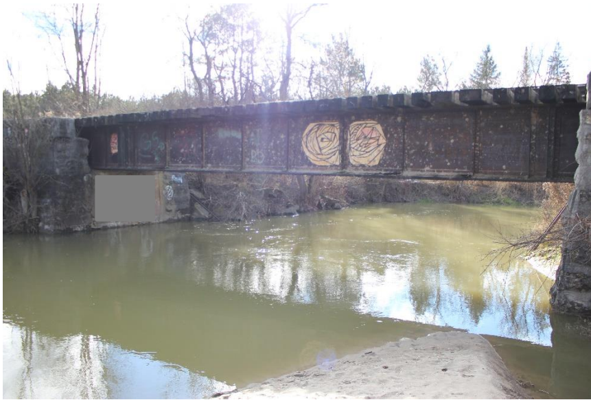
Plate 1: North elevation of the Mad River Bridge, looking south. Note: the image has been altered by ASI to block offensive graffiti.
