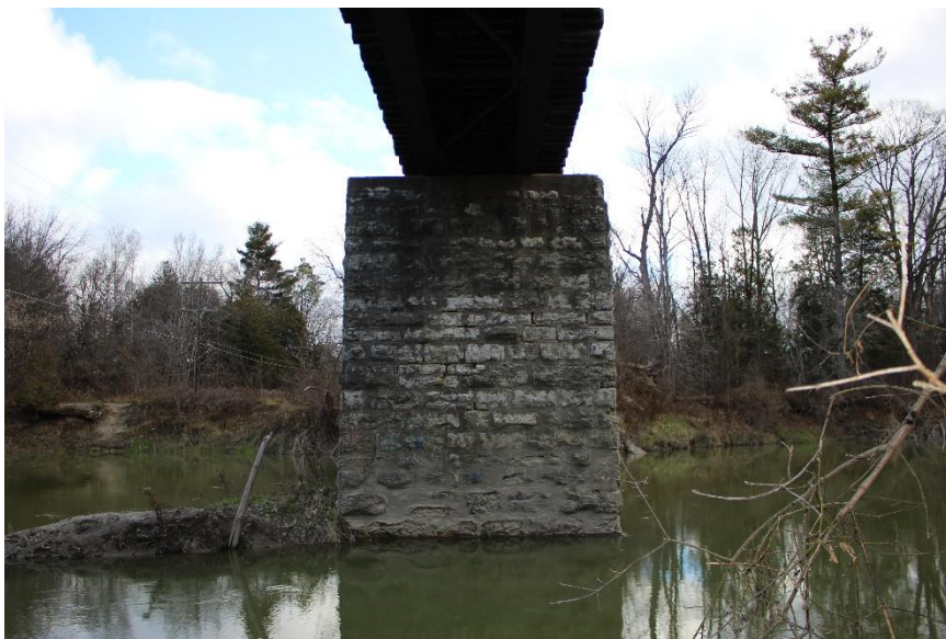
Plate 28: West face of the west pier, looking east. Note the deteriorated concrete or gunite parging.
