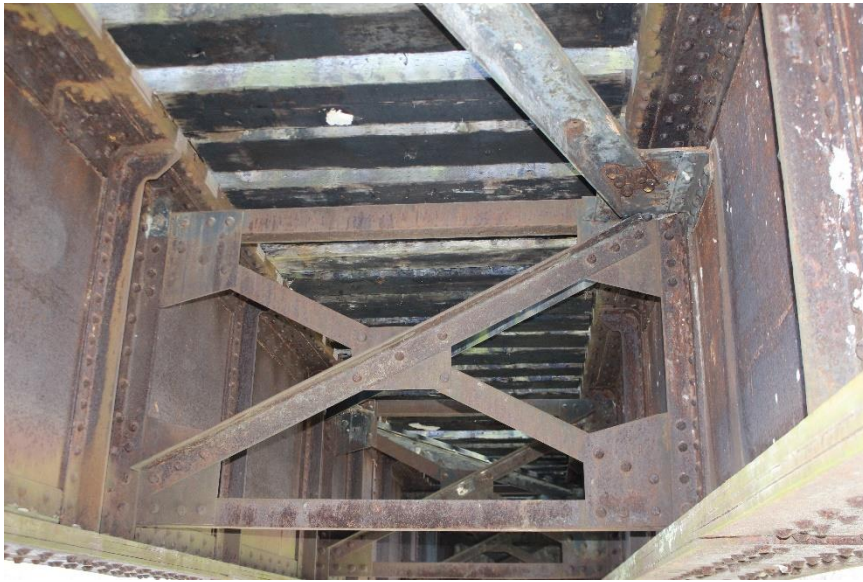
Plate 7: Riveted structural steel connections in the superstructure, looking east from the west abutment.
