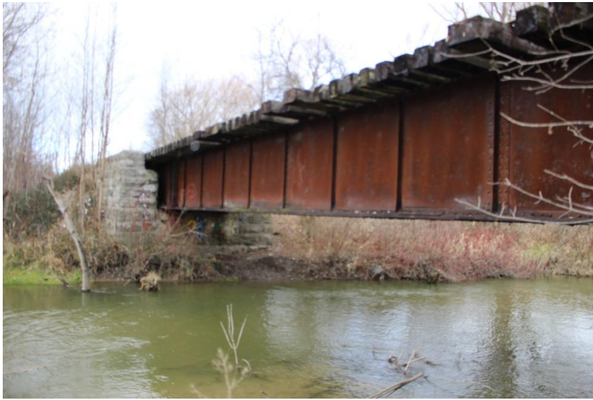
Plate 13: Oblique view of the north elevation and the east abutment, looking southeast.
