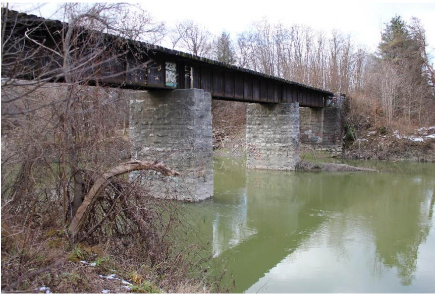
Plate 24: Oblique view of the north elevation and the east elevation of the piers, with the west abutment at rear right, looking southwest.
