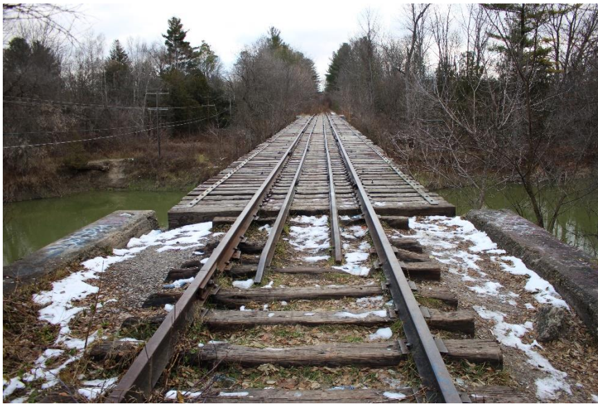
Plate 30: The bridge deck, looking east from the west approach. Note the timber ties, rail track, and bridge rails at deck level.
