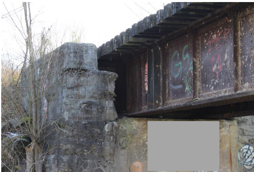
Plate 4: East abutment plate supporting the superstructure, looking southeast. Note: the image has been altered by ASI to block offensive graffiti.
