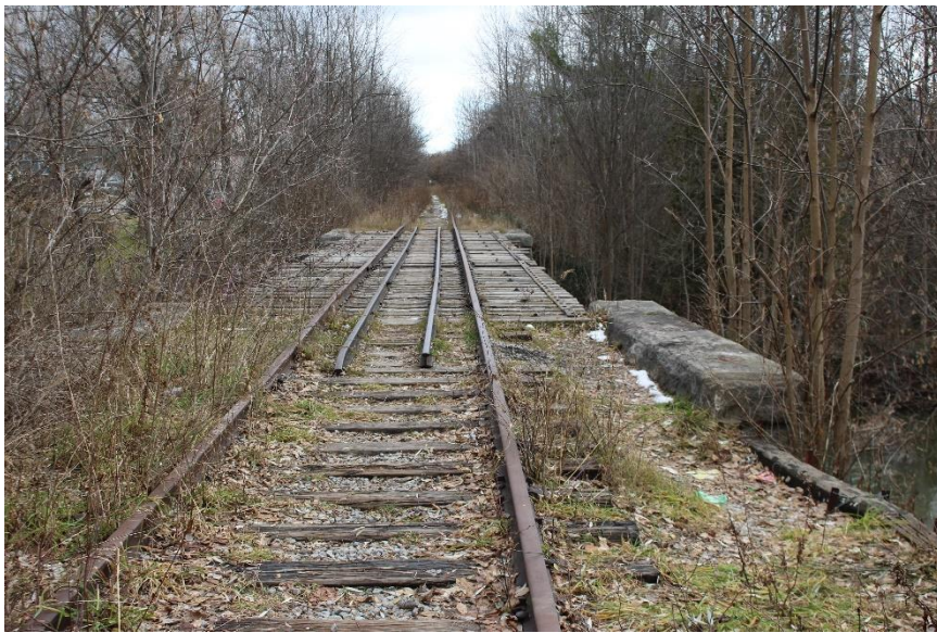
Plate 18: Open bridge deck with timber ties, rail track, and single bridge rails, looking east from the west approaches. Note the south wingwall of the west abutment and timber retaining wall at near right.
