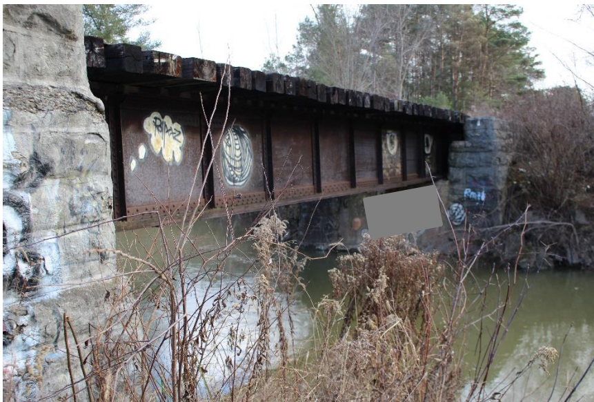
Plate 2: Oblique view of the south elevation, looking northeast. Note: the image has been altered by ASI to block offensive graffiti.
