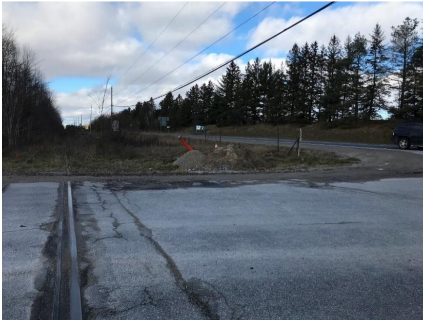
Plate 11: View of the former rail line from Sunnidale Tosorontio Townline, looking northwest, with Brentwood Road also in the photograph.
