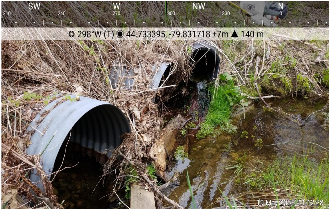
Photo 1: Twin csp inlet with discharging HDPE pipe and sediment accumulation.
