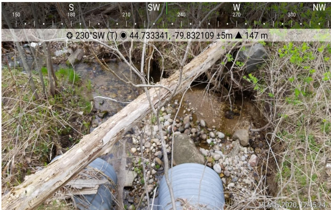
Photo 8: Continued bank erosion at the culvert outlet due top high flow events.
