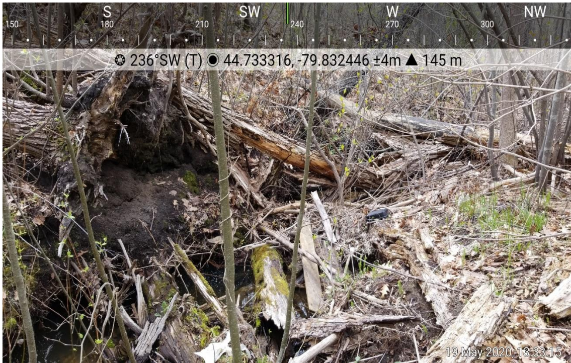
Photo 11: Multiple woody debris dams were noted within the downstream, impeding fish passage.
