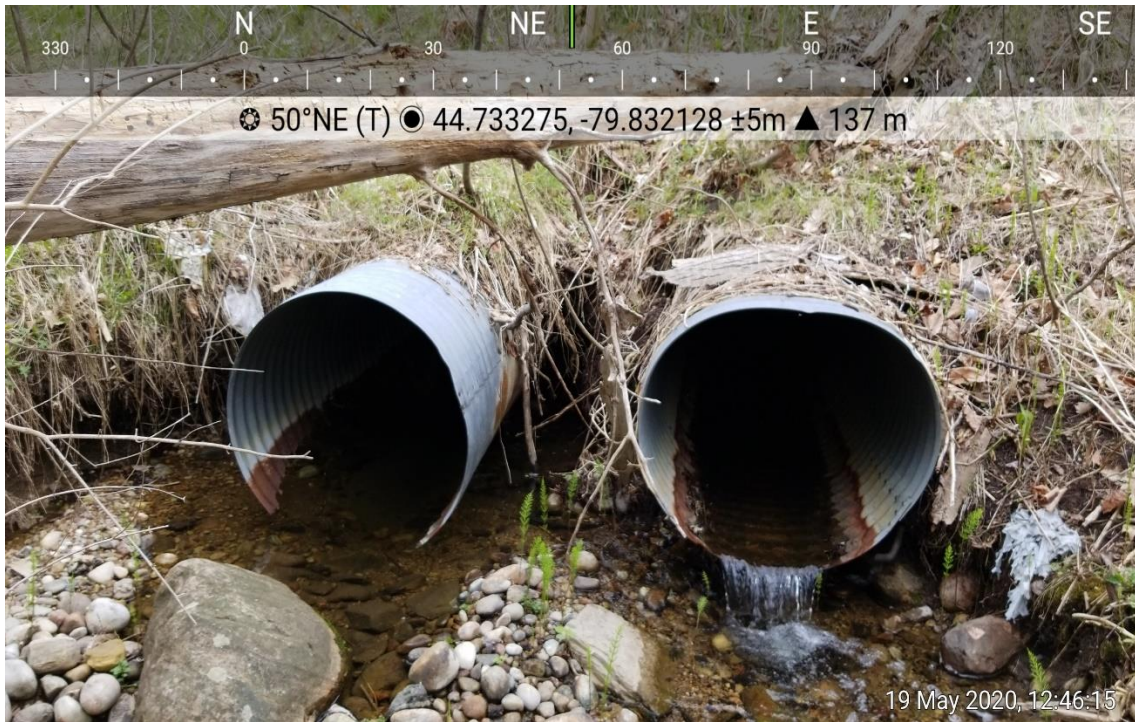
Photo 7: Perched culvert outlet with cobble and gravel accumulation.
